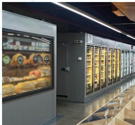
Walking Chiller Room
